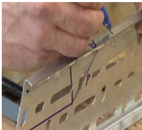
Figure 4.3 (sample Picture) Marking on the Cable Tray
