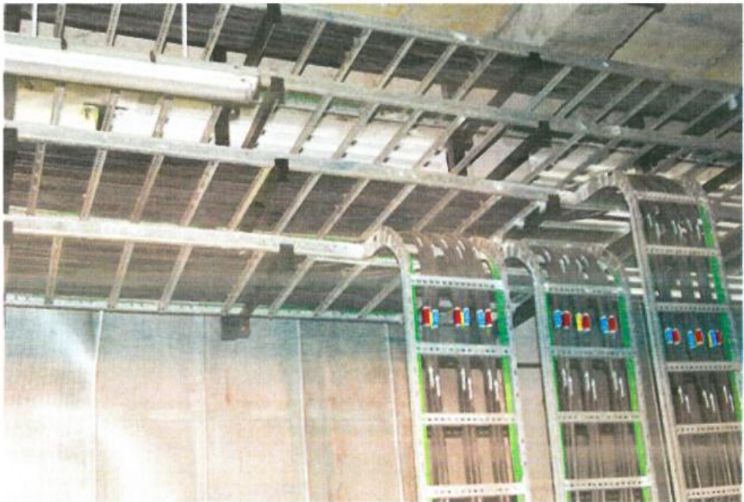
Figure – 24 (Sample Pic) Horizontal & Vertical Cable dressing
