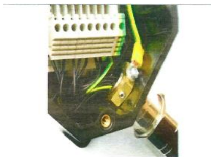
The figures presented, shows the earthing of cable gland in different ways.
