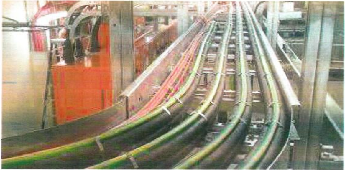
Figure – 18 (Sample Pic) Cable Dressing with Earthing Cables
