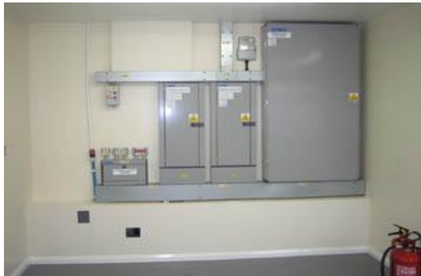
Sample Figure – 6 (Trunking Around Distribution board)
