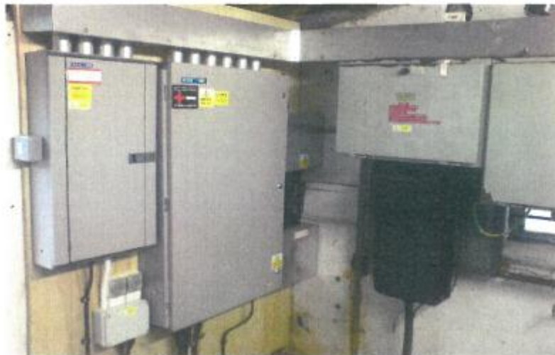
Sample Figure – 8 (Trunking Around Distribution board)
