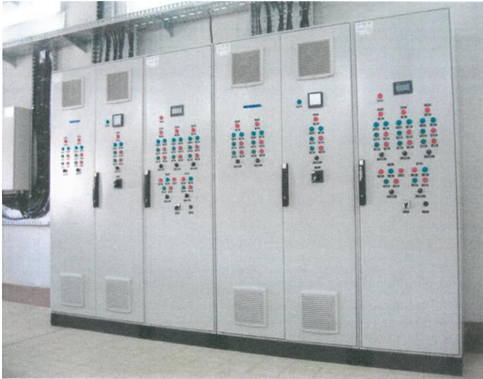
Sample Figure 7: MCC Panel Installation
