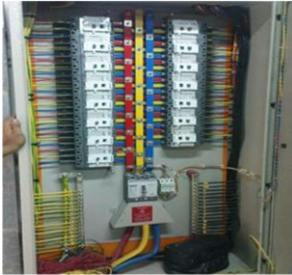
Figure - 4 (Sample Picture): Installed SMDB (Cables Terminated)
