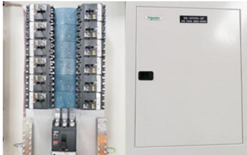
Figure - 5 (Sample Picture): Installed SMDB
